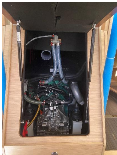
Compact – Poor ventilation
